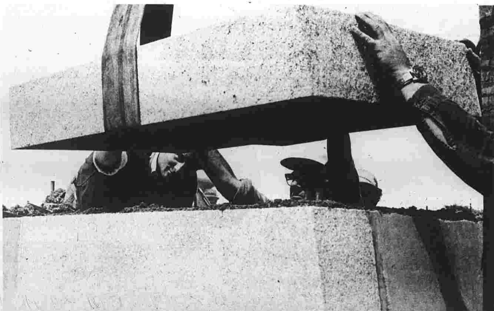
Granite cap completes a bridge on ramp where Gould's Pond used to be.
