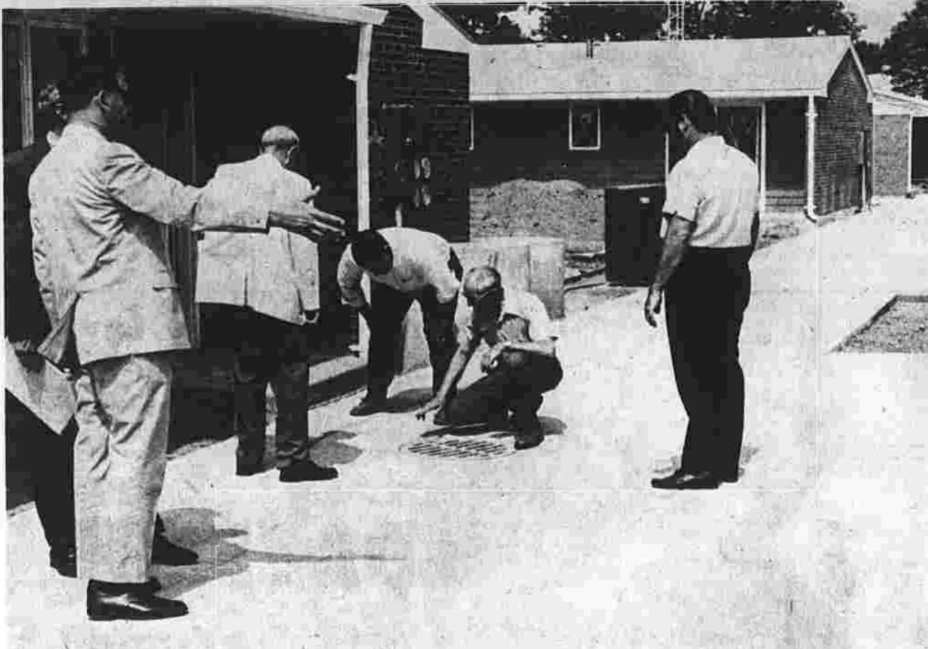
MHA members and the contractor's representatives view concrete walls at Mayfair Gardens, which the architect has called deficient and is seeking to have replaced.
